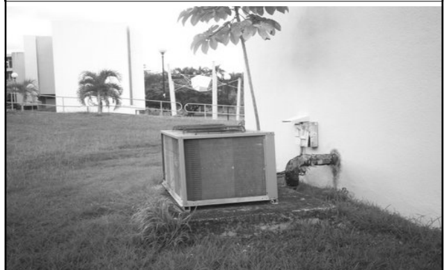
Ground Level A/C's, Power Sources, Up And Down Stairwells
